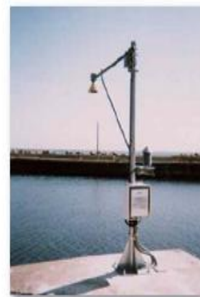
◆ Acoustic Type Gauge Station
