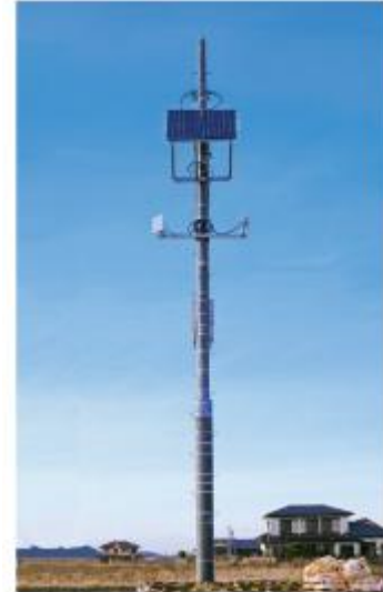
Figure 16: Costal tsunami monitoring system
