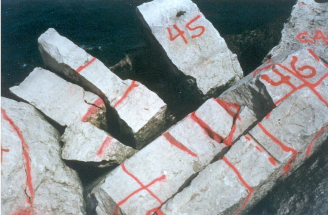
Figure V-2-13. Cracked stone - - Cleveland East breakwater, Ohio, 1990. Note continuing degradation compared to 1989 (stone is dolomitic limestone)
