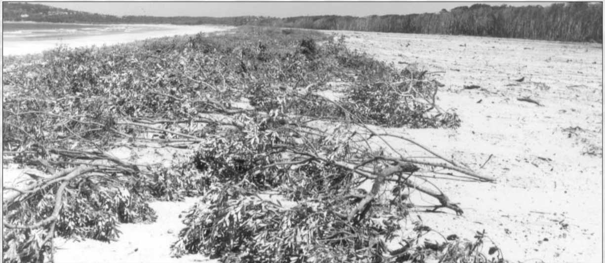
Brush matting being used to stabilise the sand surface and to initiate the dune building process by trapping wind blown sand.
