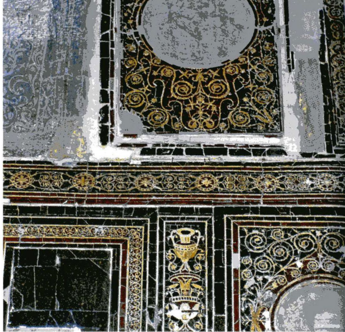
38 The wall of the Baptistery narthex , showing the remains of the original opus sectile revetment: colourful marble mosaics from the fifth century.
