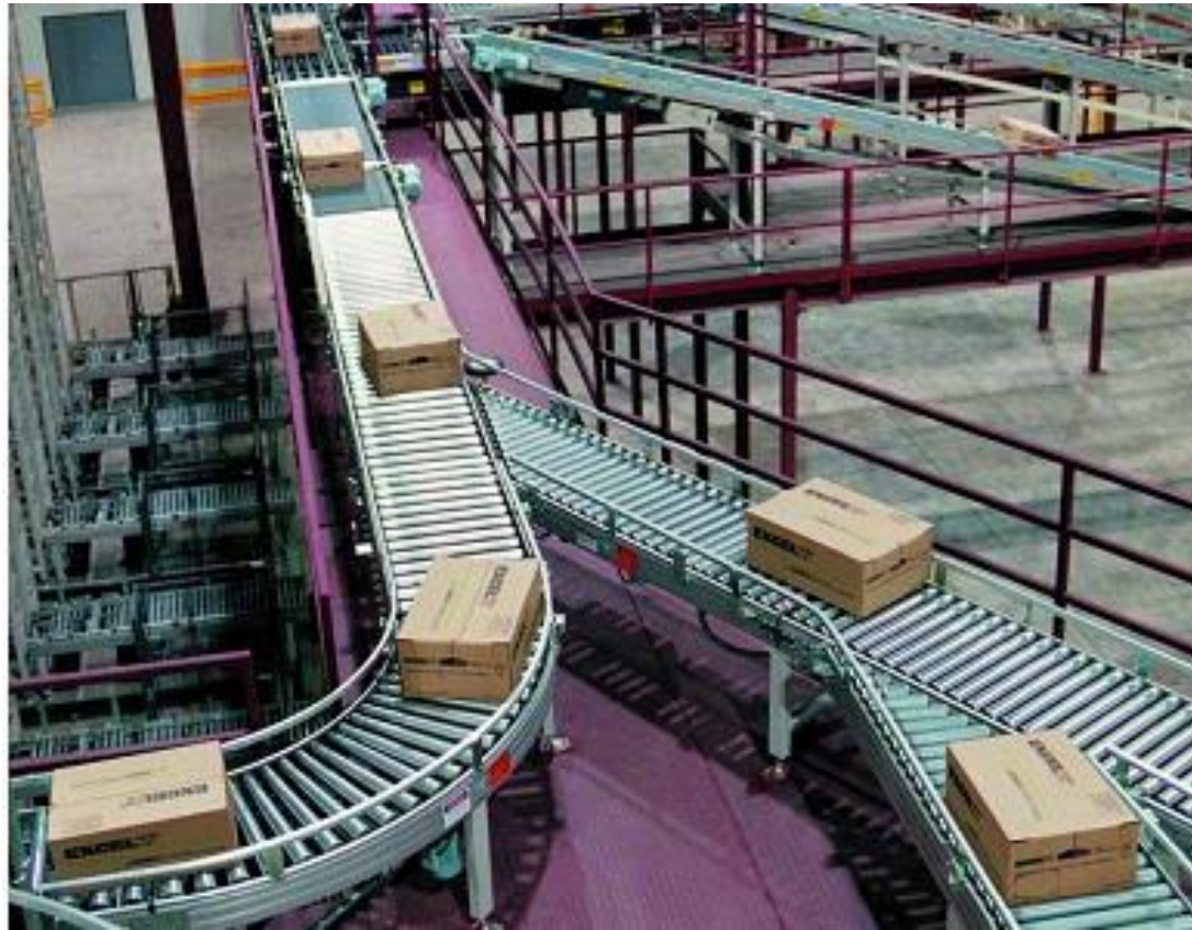
Conveyors in sloping with rollers "idle"
