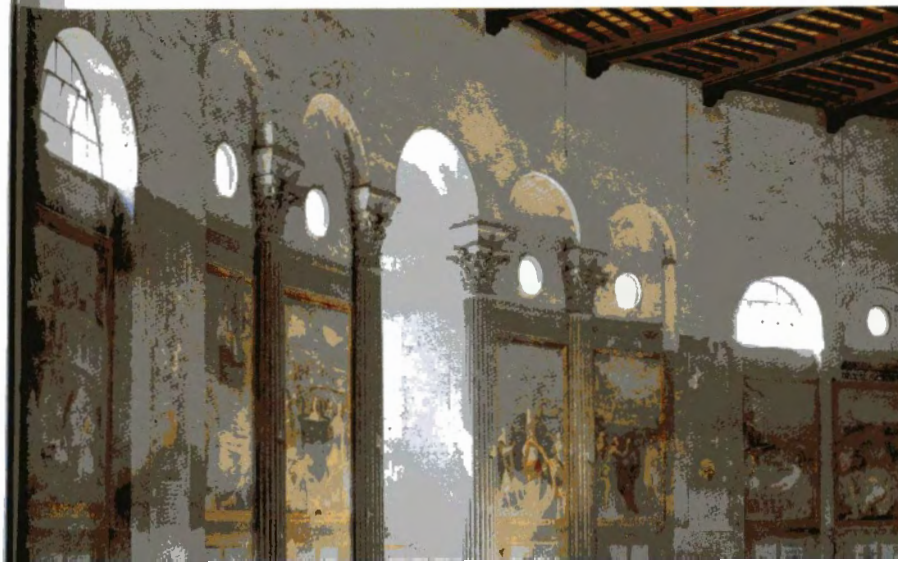
108 Four spolia columns with fluted marble shafts and Corinthian capitals (late third century). The columns are set into the outer wall of the church, but they originally separated the ambulatory from the south-western narthex which was removed in the fifteenth century when the church was rebuilt in a reduced form. The capitals probably come from the same source as the set of twenty-four in Santa Sabina 10 [101].
