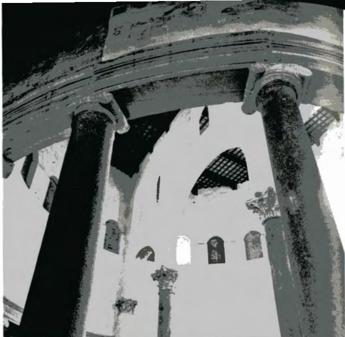
104 Arcade supported by two huge spolia columns with grey granite shafts and Corinthian capitals. The arcade was built during the reign of Pope Innocence II (1130–1143) to reinforce the high walls of the central chamber which were in danger of collapsing.
