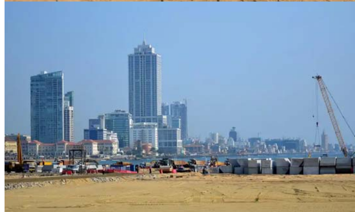
Reclaimed sand is sprayed at the construction site for Colombo International Financial City, Sri Lanka; a general view of the construction site; a sign at the site
