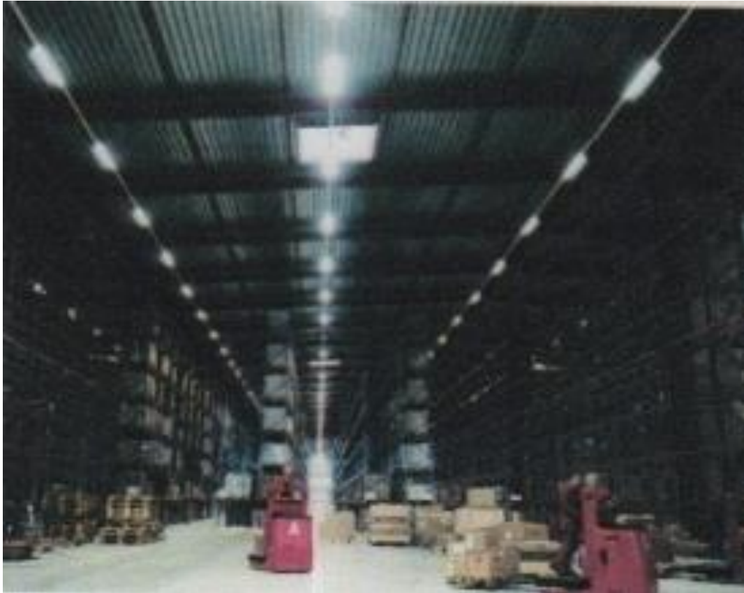
Lighting lines of lighting fixtures with fluorescent tubes
