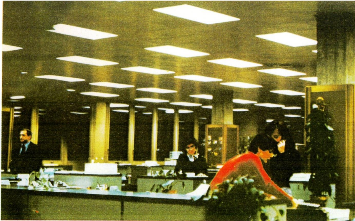
Lighting fixtures with fluorescent tubes in a shoe factory
