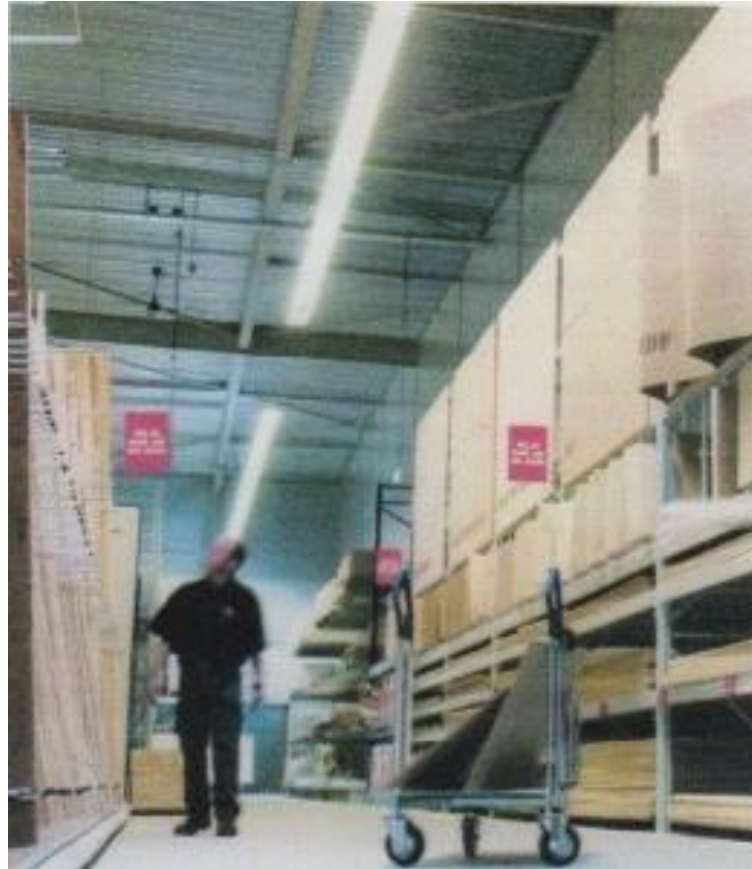
Lighting lines of lighting fixtures with fluorescent tubes
