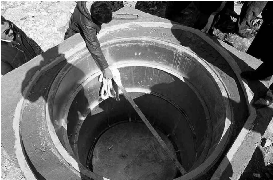
Fig. 7.40 Interior of a seismic vault made of welded metal sheets. The vault is big enough to accept weak- and strong-motion instrumentation together with data acquisition and transmission equipment.
