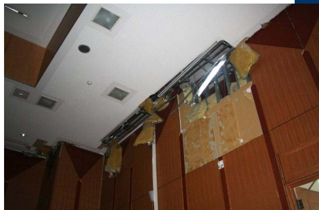
(b) Fall of ceiling of Municipal Assembly Hall (1)
