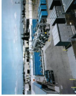
Fuel Cell Energy 2 MW MCFC
