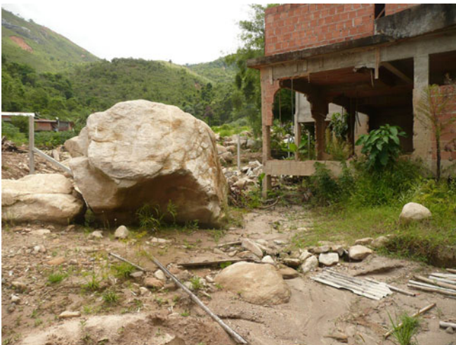
Fig. 30 Debris flood damage during the January, 2010 flooding at Teresopolis in the Serrana Region, Brazil. The large boulder was rolled by a 2-m deep flow, but the concrete structure on the right was only partly damaged (Photo by O. Hungr)
