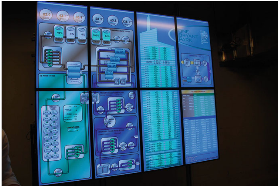
Fig. 7.17 Control system, © photo by the author
