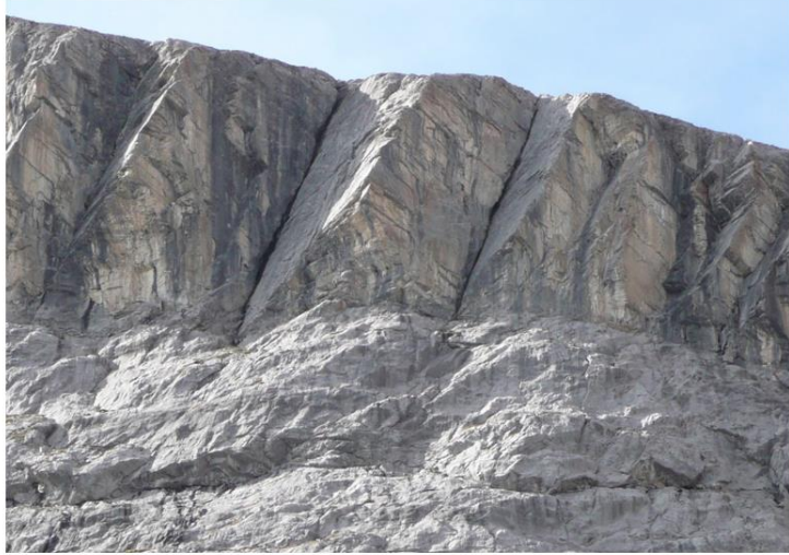
Fig. 8 Scars of wedge failures in limestone, Canmore, Alberta, Canada. The cliff is approximately 50 m high (Photo by O. Hungr)
