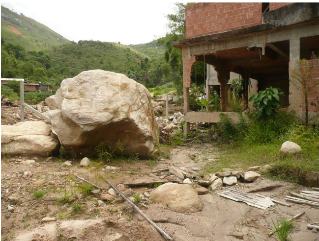
Fig. 30 Debris flood damage during the January, 2010 flooding at Teresopolis in the Serrana Region, Brazil. The large boulder was rolled by a 2-m deep flow, but the concrete structure on the right was only partly damaged (Photo by O. Hungr)
