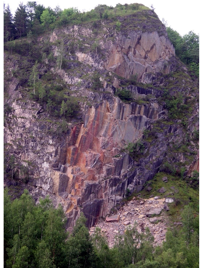
Fig. 4 Block topple in limestone, Czech Republic (Photo by O. Hungr)
