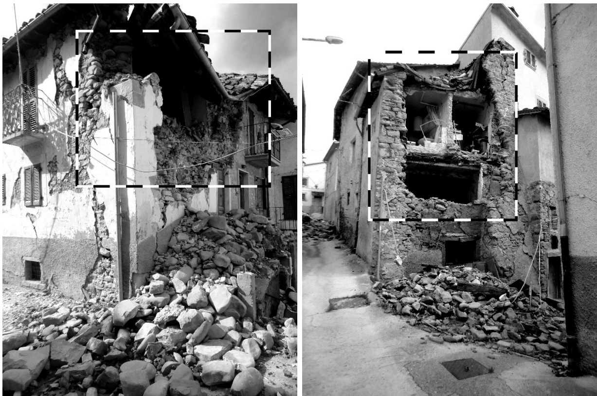
Figure 10: out-of-plane overturning of the perimeter wall (Accumoli).
