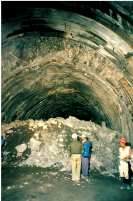
Figure 24: Large displacements in the top heading of the headrace tunnel of the Nathpa Jhakri Hydroelectric project. These displacements are the result of deteriorating rock mass quality when tunnelling through a fault zone.
