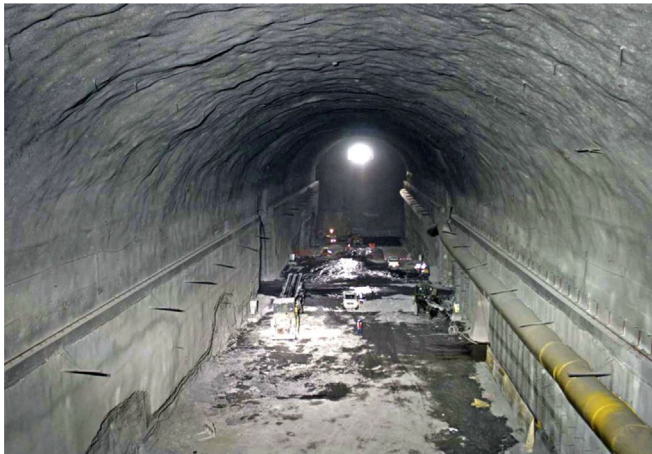
Fig. 24. The 26 m span, 50 m high Ingula underground powerhouse cavern after excavation of bench 3. Photograph provided by G. Keyter and reproduced with permission of ESKOM South Africa.
