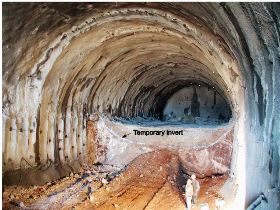
Figure 15. Top heading and bench excavation in a weak rock tunnel where a temporary shotcrete invert was used to control floor heave.
