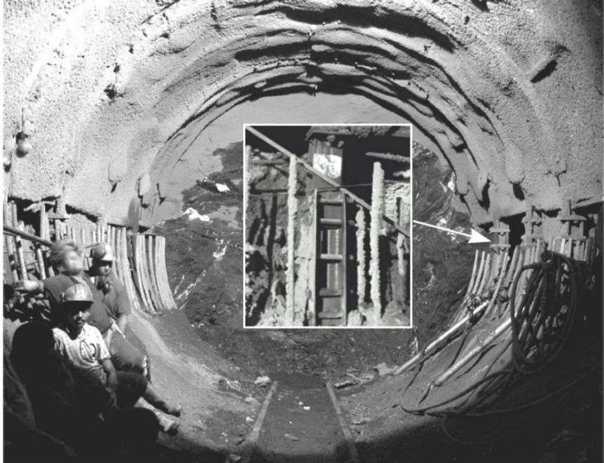
Figure 31. Initial Liner composed of circular steel arch and 20 cm of shotcrete. Inset shows detail of sliding joint with shotcrete gap. Note rebar in place to reinforce final shotcrete layer.
