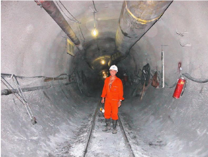
Figure 39. Completed section of tunnel with a 60 cm thick reinforced shotcrete lining, placed in two layers as described above.
