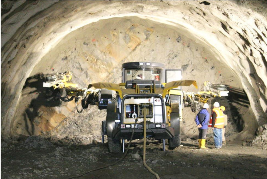
Figure 9. A simple top heading shape in good quality interbedded sandstones and siltstones. The tunnel arch is supported by means of rockbolts and a layer of shotcrete and no face support is required. The flat floor requires no special treatment other than good drainage of surface water accumulations.
