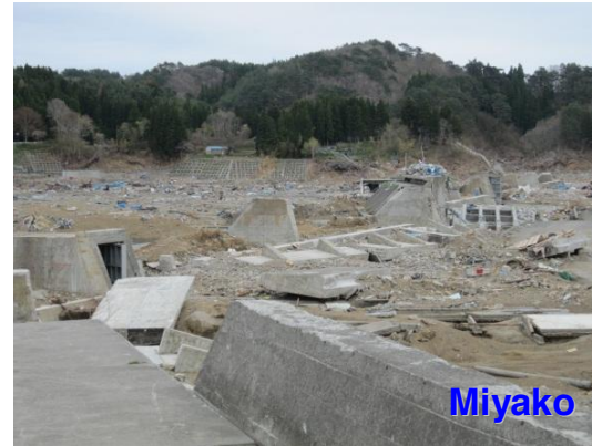
The 10m-high seawall was destroyed in Taro district, Miyako city, Iwate Pref.
