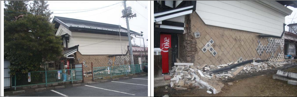
Photo 8: Fall of exterior mud finishing of traditional ware house walls
