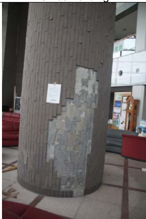
(c) Fall of finishing tiles on a column
