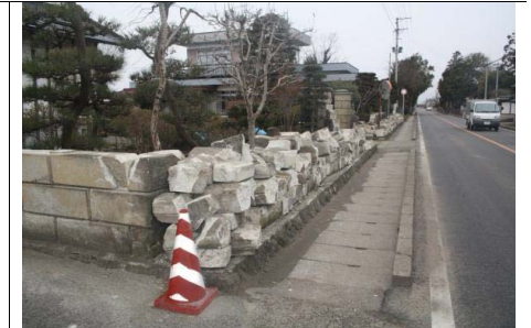
Photo 5: Fall of masonry walls
