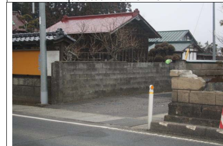
Photo 6: Undamaged concrete block walls and damaged masonry walls
