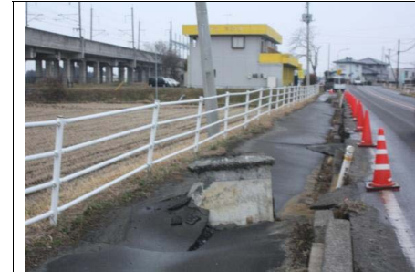
Photo 4: Lifting of a man hole due to soil liquefaction near Shiwahime
