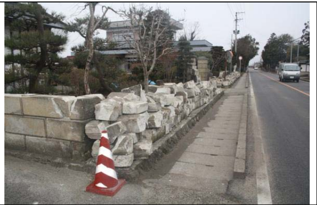
Photo 5: Fall of masonry walls
