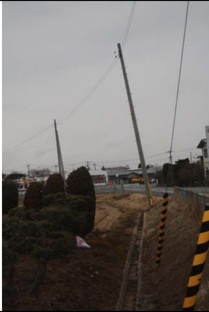
Photo 13: Tilting of utility poles
