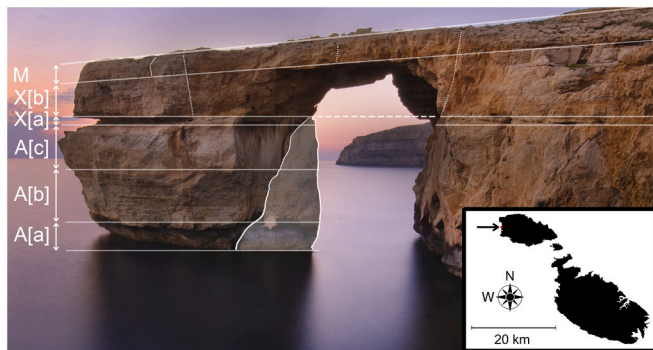
Fig. 2. Lithology of the Azure Window, after Pedley (1978). Labels ‘A’, ‘X’, and ‘M’ denote Attard, Xlendi and Mara members respectively. Letters in square brackets denote principal subdivisions of facies. Dotted lines denote visible cracks on the Xlendi and Mara members. The horizontal, dotted line underneath the bridge marks the boundary above which rockfall (largely from the X[b] member) took place since a c. 1900 photo by Richard Ellis (Panel (a) of Fig. 3). The shaded region on the pillar marks a large section that collapsed in 2012. The inset shows a map of the Maltese Islands with the location of the former Azure Window (west coast of Gozo), marked with an arrow. The site coordinates are 36°03’12.9”N, 14°11’19.1”E. (Image copyright: J. Caruana.)
