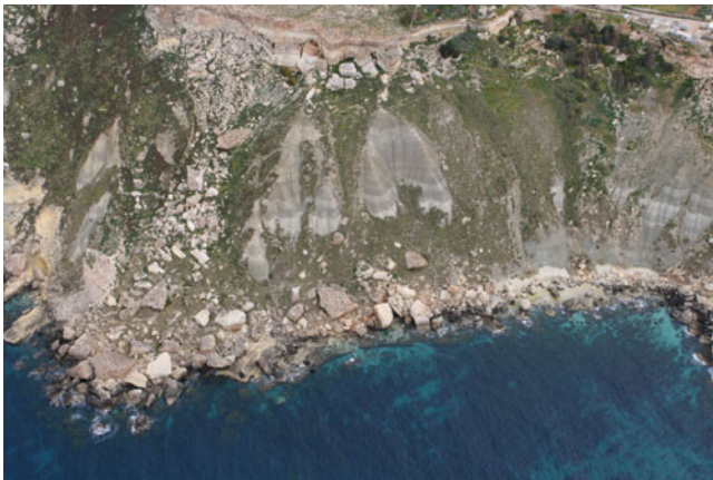
Fig. 4 Evidence of rock falls occurring along the north-western coast of Malta (Courtesy of Ten. Col. M. Marchetti)
