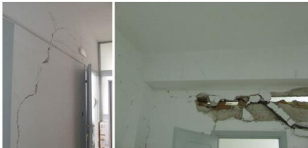
Fig. 10 Damage on non-structural elements along the X2 frame at the ground and first storeys
