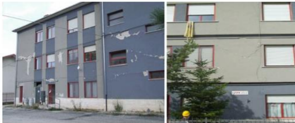
Fig. 9 Damage on infill panels along the X1 and X3 Frames
