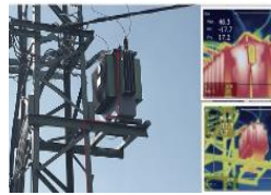
Advanced concept of efficient use of transformers leveraging the DTR technology (Applied)
