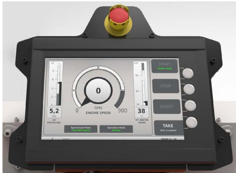
Fig 14-2 Local operator panel
