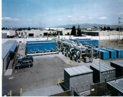
Fuel Cell Energy 2 MW MCFC
