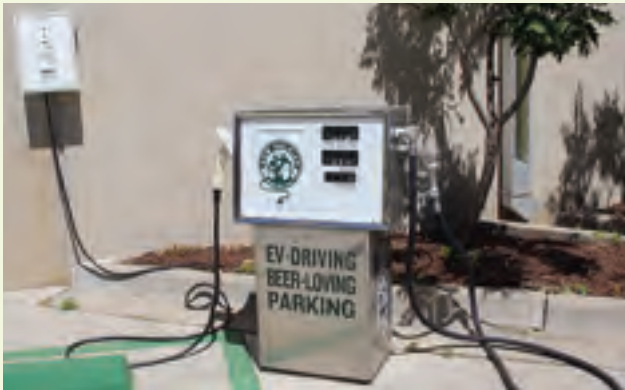
Providing electrical charge points for customers and staff from rooftop solar. PHOTO: A MELCK
